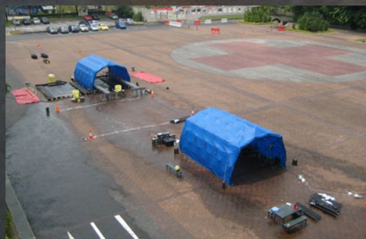
A typical MRF Deployment Set-up using the Deployable Rapid Assembly Shelter (DRASH)
