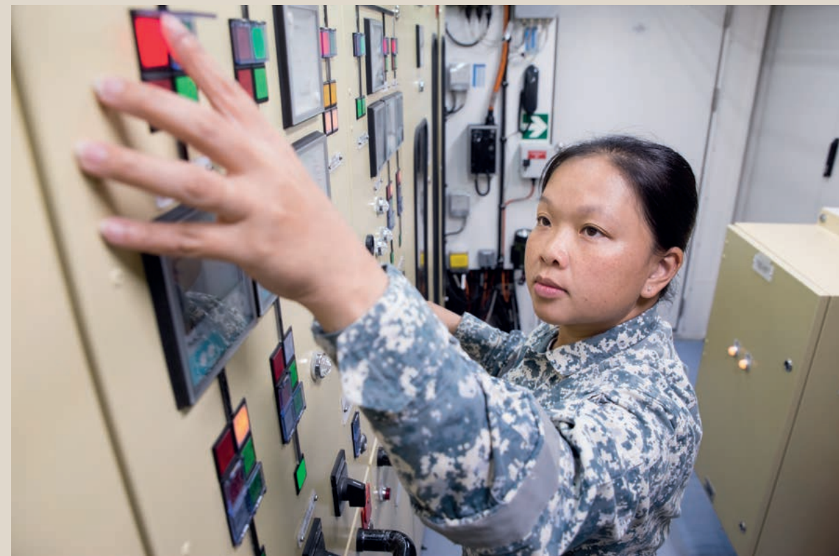
ME2 Michelle Mok conducting a system check on one of the main switchboards on board the littoral mission vessel, Sovereignty , expected to be commissioned in 2017. The engineering systems on board the littoral mission vessels are automated.
