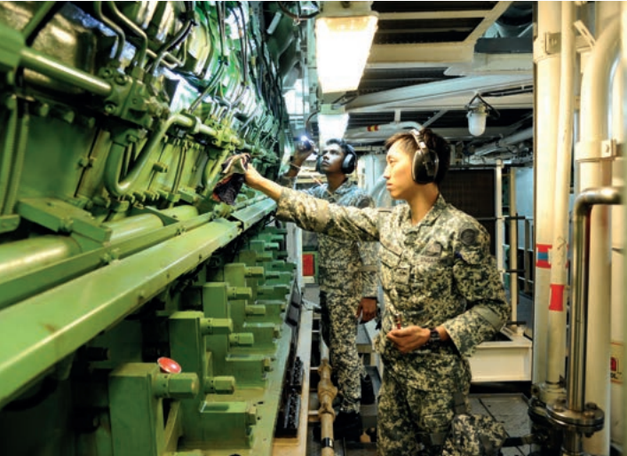
Marine Systems Operators conducting routine checks on RSS Steadfast's engine in the Engine Room. Engineering crews aboard RSN ships are crucial in maintaining the health of all engines and machinery.
